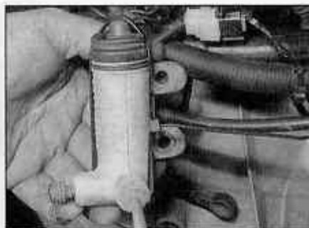
4.7 Fit a cable tie around the clutch slave cylinder to prevent the piston coming out
